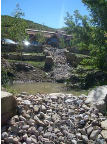
Picture 7: Silver Star Wet Detention Basin and Gabion.
