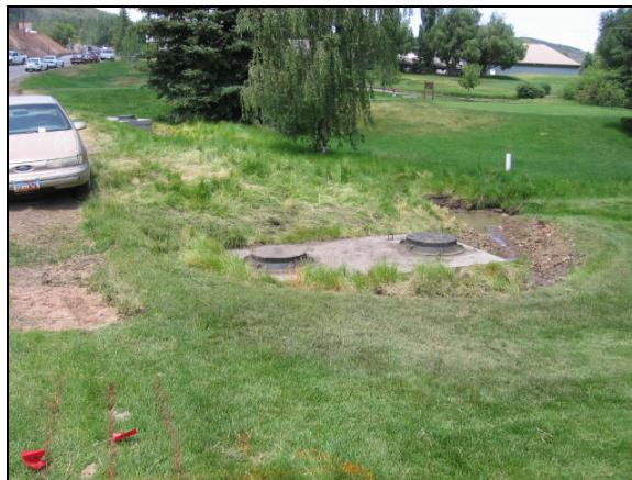
Picture 12: Silver Star Development wet vault.
