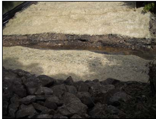
Picture 13: Silver Creek Crossing Boothill Transmission Line.
